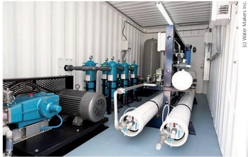
A container-desalination facility, which, powered by a GF 1000, is able to supply 75,000 litres of drinking water per day.
